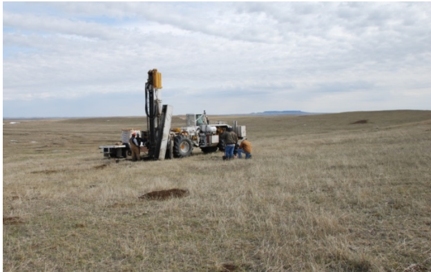
Formation Resources drilling for uranium, molybdenum, and germanium under a subsurface mineral permit in Billings County during the fall of 2008.
