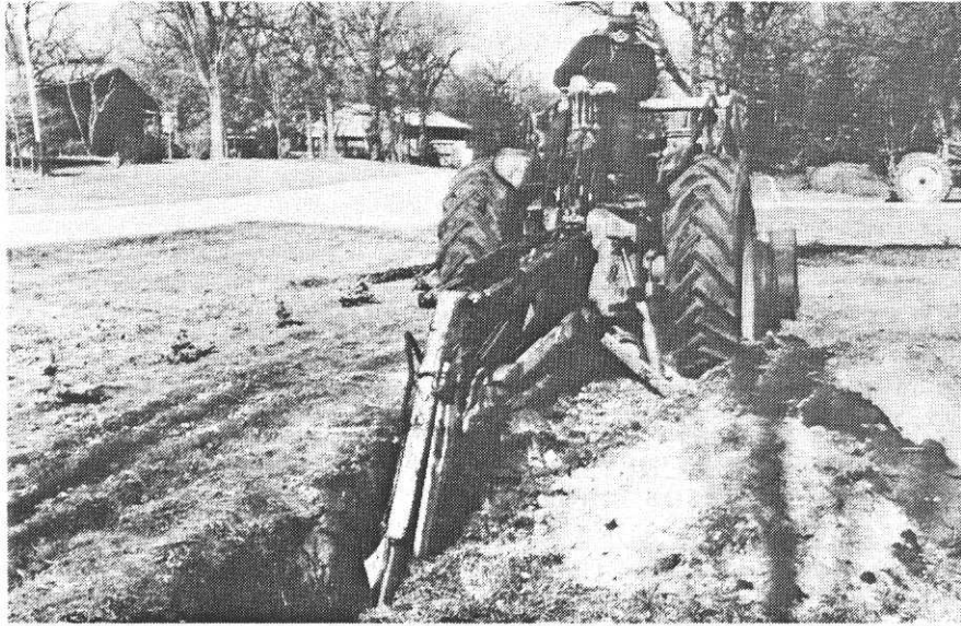
Figure 1. Representative Gordon Berg operating a backhoe, digging a trench across an old Devils Lake beach. This trench was dug in the Lakewood area.
