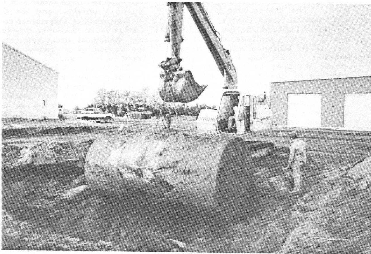
Figure 1. Oil tank being lifted from excavation near Plant Services complex, UND campus.
