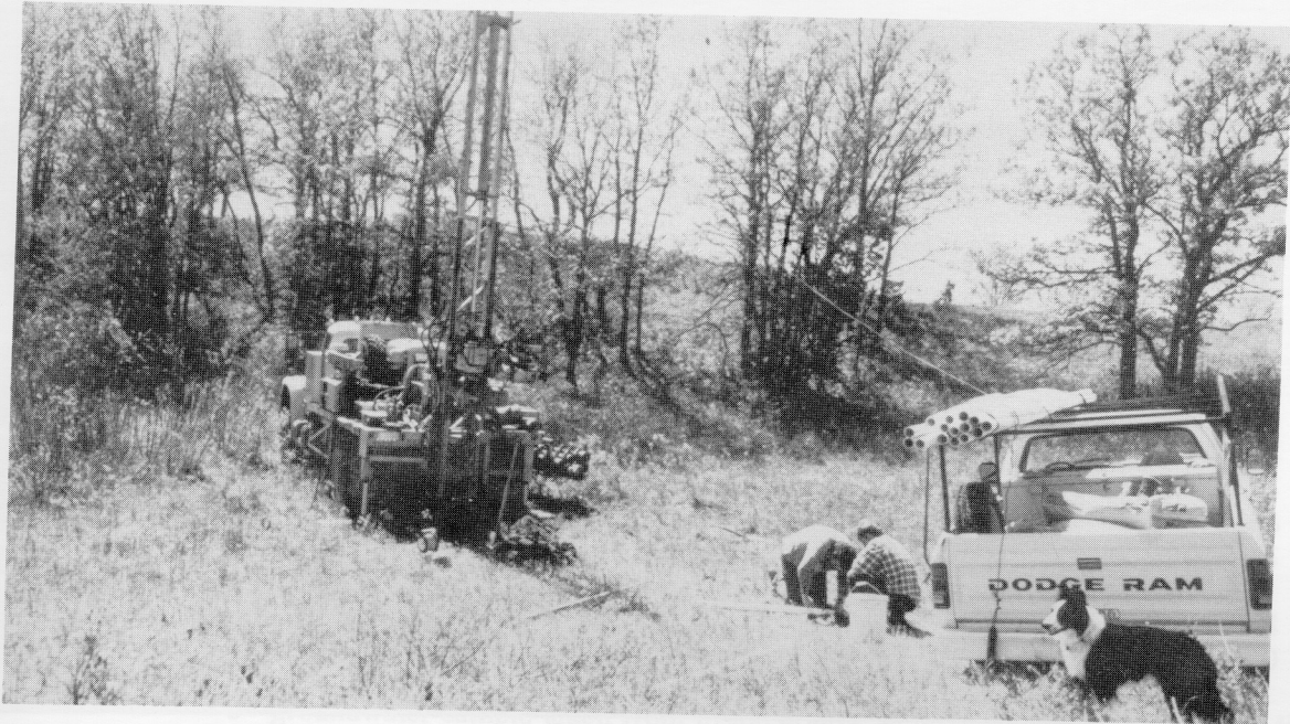
Figure 6. Installing monitoring well 2 at the well 2 and 3 nest. View is to the southwest.
