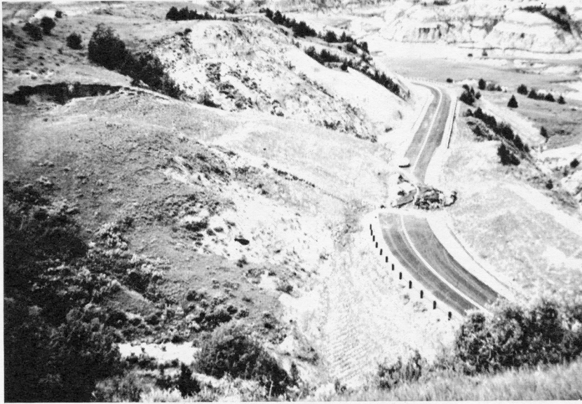
FIGURE 2. Landslides in South Roosevelt Park caused by inadequate understanding of geologic factors involved in construction in this area.
