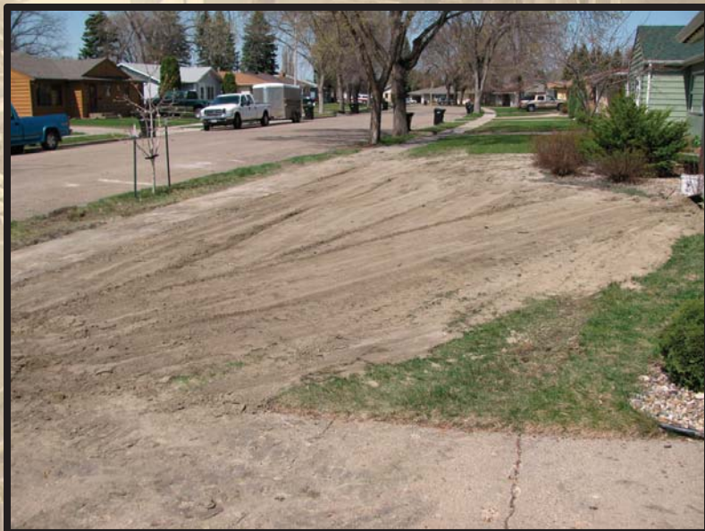
Figure 4 (left). The completed well field. Drill cuttings and other debris were removed and the surface smoothed and regraded. Copious amounts of topsoil and compost were required to recondition the soil before reseeding the lawn.
