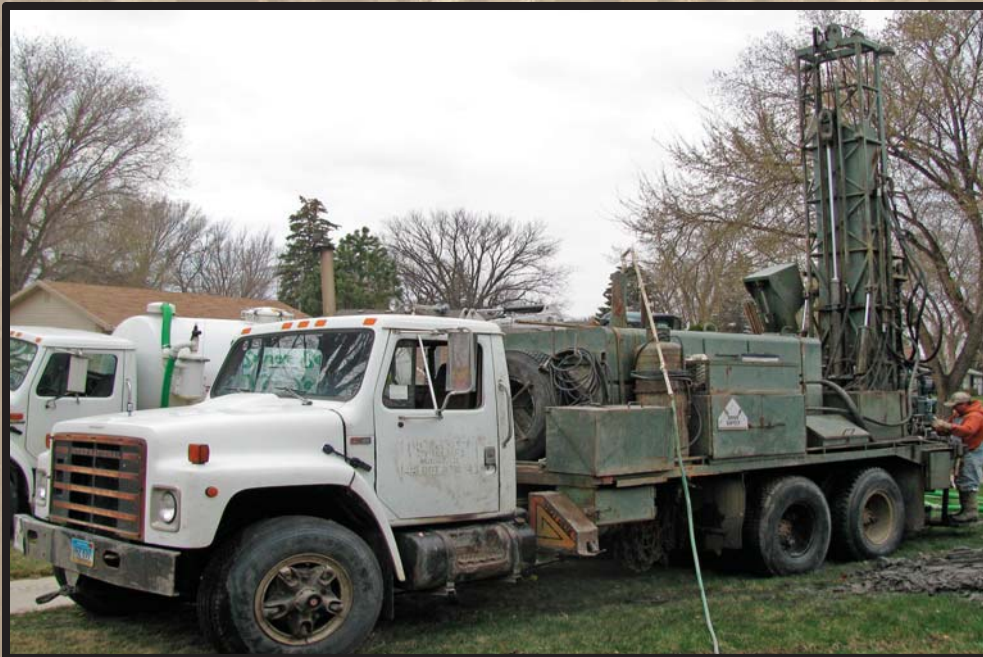
Figure 1. Drilling the wells. Space was tight, even in the front yard, as these pictures show. The truck-mounted drill rig remained within our property lines throughout the entire drilling operation, and although the grass suffered under its weight the adjacent sidewalk was undamaged.
