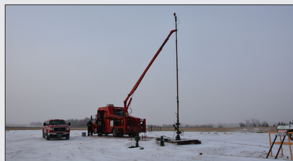
Figure 3. Slickline unit set up over NDIC Well # 12363, Astrid-Ongstad 14-22 north of Tioga, ND.
