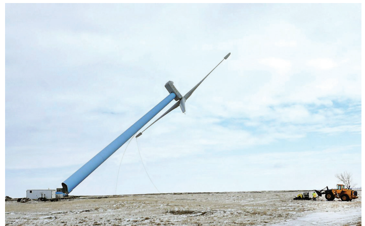
FIGURE 4. Decommissioning of the first wind towers in North Dakota south of Minot. This process is called chop and drop, similar to felling a large tree, where the base of the tower is cut and the tower is pulled over with cables and heavy equipment (Image by Jill Schramm, Minot Daily News).
