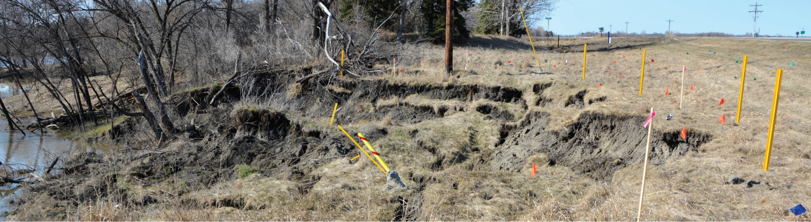
Riverbank slumping along a cutbank meander of the Wild Rice River encroaches into the utility and transportation corridors adjacent to South University Drive, south of Fargo (NDGS, 2022).
