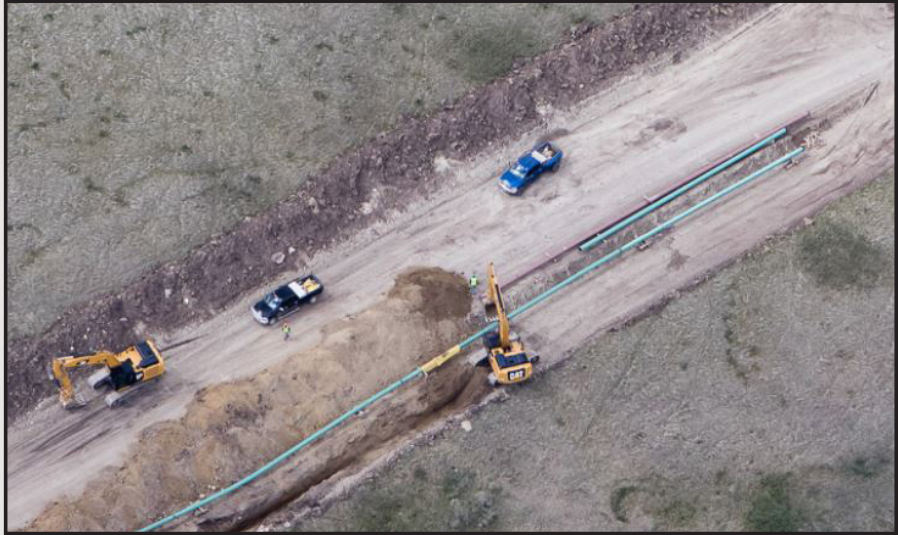
Figure 3. Installation of new oil gathering pipeline near Stanley. Photo courtesy of Vern Whitten Photography (2016).
