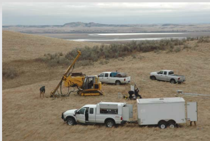
Figure 2. Drilling and installation of one of the monument braces for the new PBO GPS station near the Stumpf Natural Area southeast of Huff, in eastern Morton County, south-central North Dakota. Components installed include a high-precision GPS receiver and antenna, along with power and data communications equipment, housed in a weather-tight enclosure.
