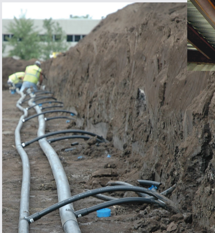
Figure 4. The two pipes running parallel to the trench wall are the supply and return headers. Fluid from the heat pumps travels along one and is delivered to every ground loop in the circuit (the pairs of small-diameter pipe sticking out of the ground) then returns to the heat pumps via the second header. Note that all the ground loops are connected to both. And your eyes are not playing tricks on you: the header pipes really are different sizes. It is a way of ensuring that the required fluid flow rates are maintained throughout the closed circuit without compromising the overall efficiency of the GSHP system. The building in the background is the State Water Commission.
