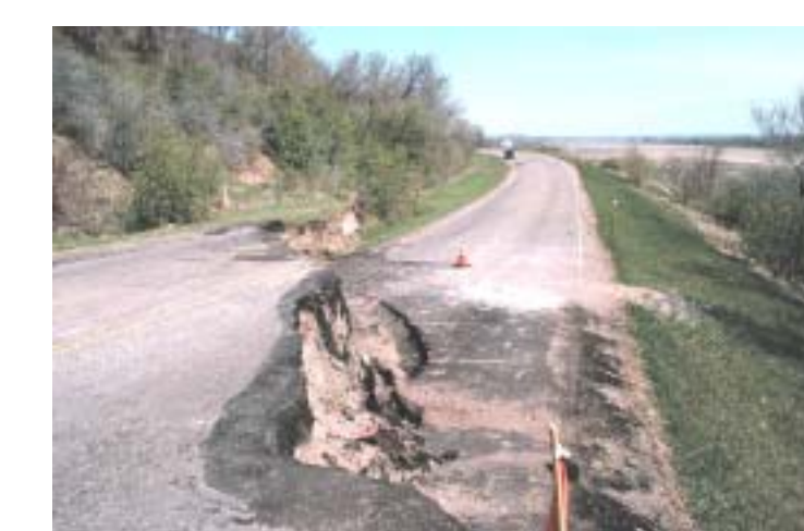
A landslide closes North Dakota Highway 1806 in 1997.
