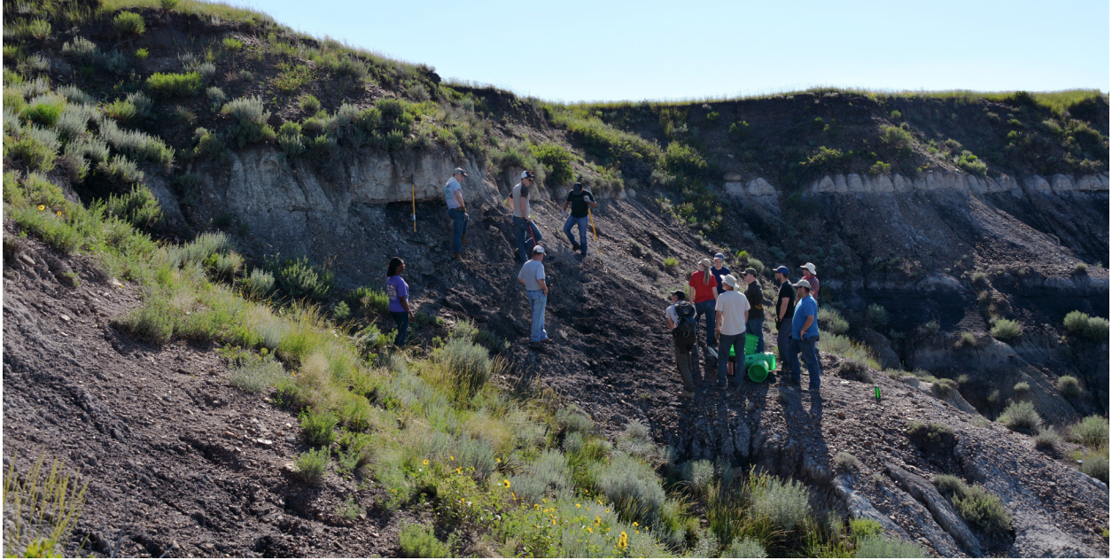
Figure 27. Staff from the University of North Dakota College of Engineering & Mines prepare to excavate the uppermost portion of the Harmon lignite in T136N, R102W, Sec. 7 in June of 2018. Although early samples of the upper few inches contained up to 555 ppm REE, the enrichment in this setting was very thin and slight, likely because REEs were mobilized during relatively low-intensity weathering of the overlying Quaternary terrace.
