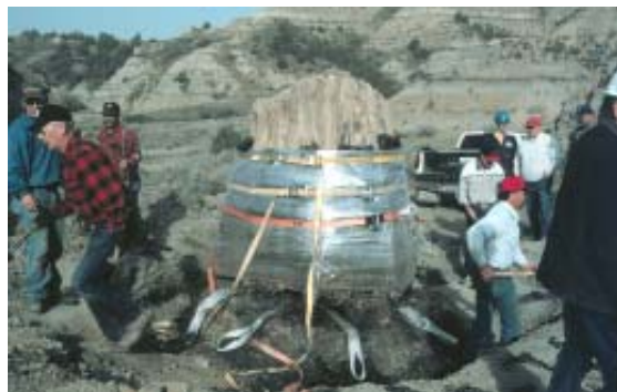
Preparing petrified tree stump for removal. Note shrink wrap, strapping, and straps for lifting placed in tunnels under the stump.
