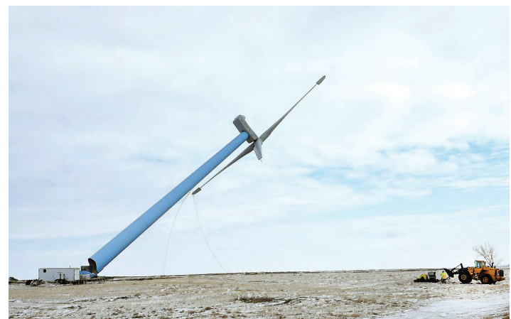
FIGURE 4. Decommissioning of the first wind towers in North Dakota south of Minot. This process is called chop and drop, similar to felling a large tree, where the base of the tower is cut and the tower is pulled over with cables and heavy equipment (Image by Jill Schramm, Minot Daily News).
