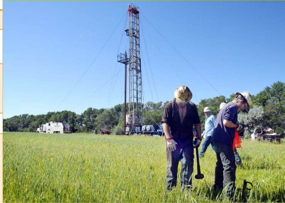
Garrett Van Dyke, left, and Jesse Zanh, both with Ham's Well Service, anchor a cable stretching to the top of the 96-foot-tall derrick and workover rig while plugging an abandoned oil well last week west of Antler in Bottineau County. Mike McCleary Bismarck Tribune
